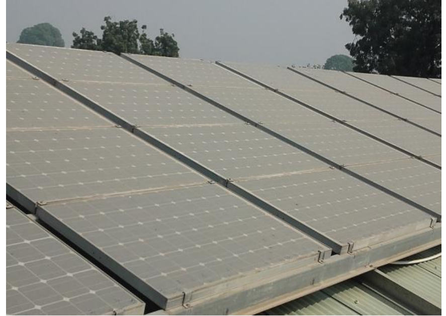
Dust and Pollution over Solar Module
